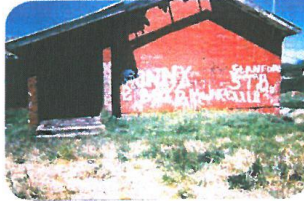
Acordia: A dilapidated toilet at the back of a school. There is no security gate and the property could be used by vagrants for illegal activities.
