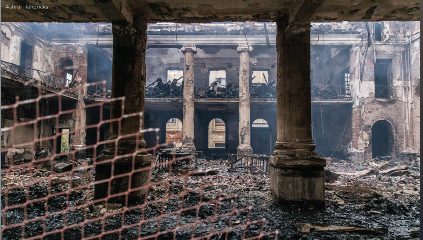
The University of Cape Town's Jagger Library, before (above) and after the fire
