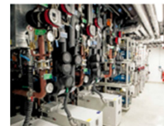
Top: A refrigeration plant in one of the buildings at Roche in Penzberg Below: The plant room for the refrigeration system
