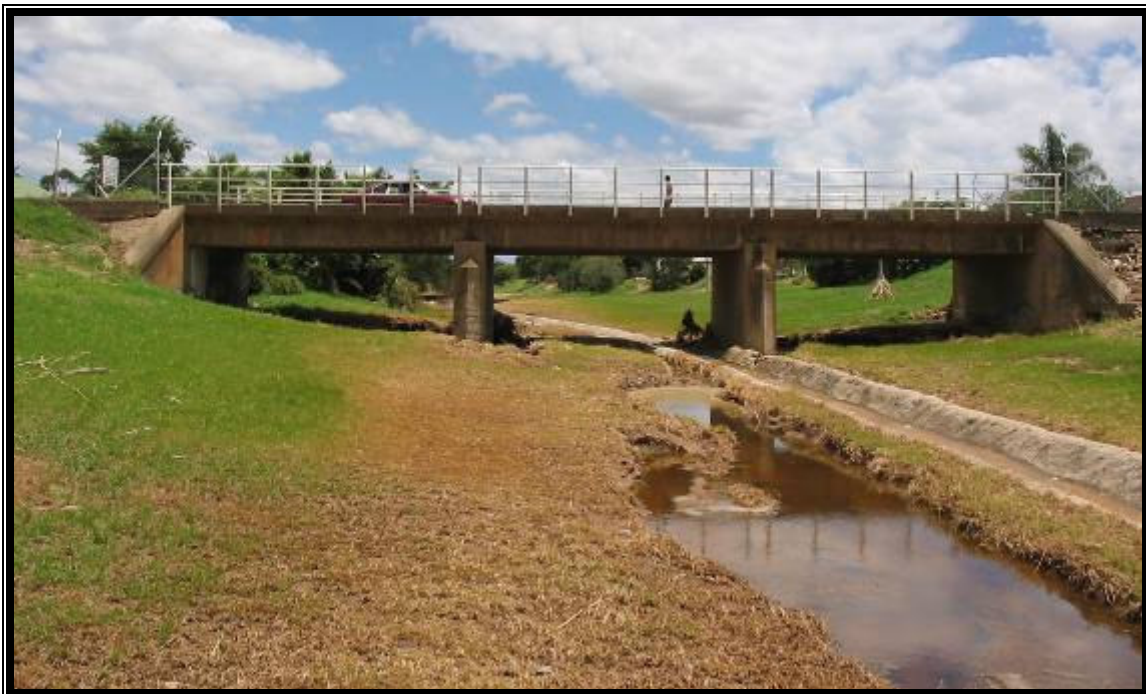
Fig 17: The same bridge as in Fig 16 above, photographed on the 28 th December 2004.
