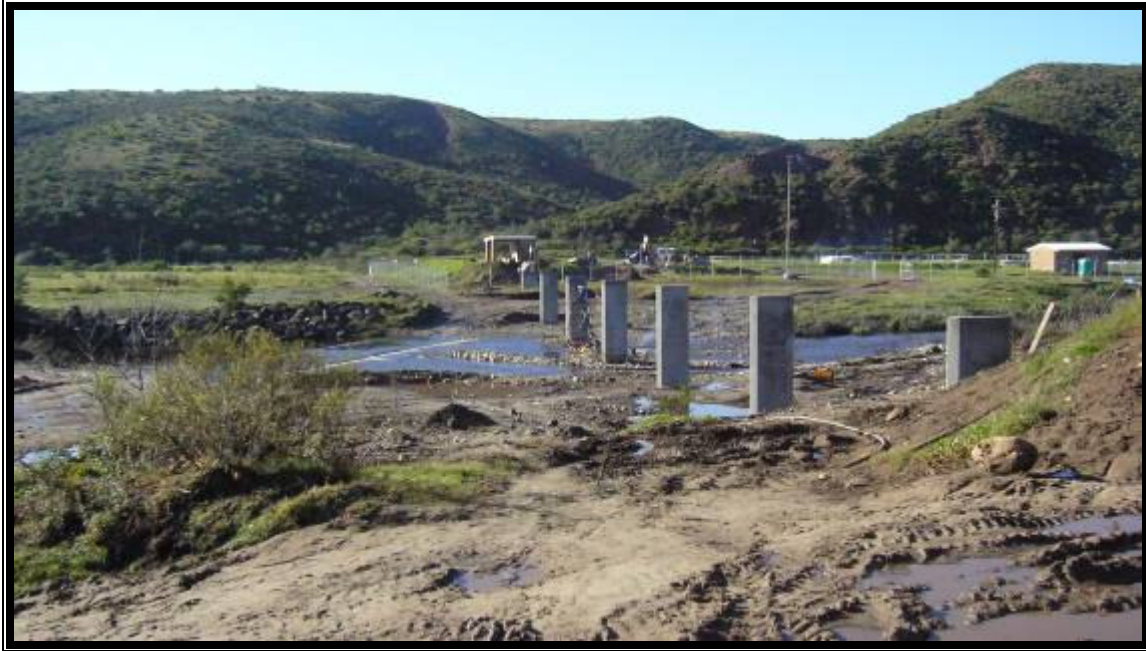
Fig 27: The reconstruction of the Heidelberg sewerage works, June 2005. The concrete pillars across the river are to carry the sewage pipeline from the Heidelberg side of the Duiwenhoks River to the opposite bank where the sewerage works are situated.
