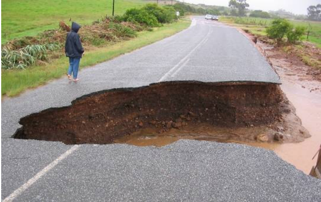
Fig 25: Damaged road near Heidelberg, Eden District.
