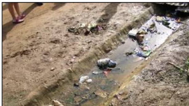
Fig 20: Shallow, debris filled stormwater drain in Suurbraak.
