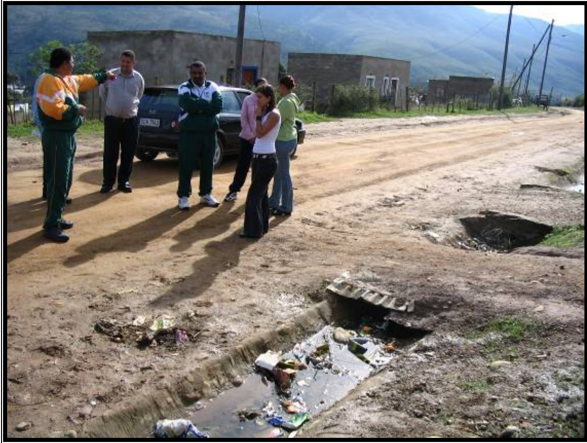
Fig 24: This picture of the low income settlement in Suurbraak shows the shallow open storm water drainage system. As well as being of an inadequate size to deal with the amount of rain typically experienced in this area, as is illustrated, these drains become blocked by litter and other debris,. This area is situated on a slope, so when the drains overflow, the water runs across the road and into the houses.
