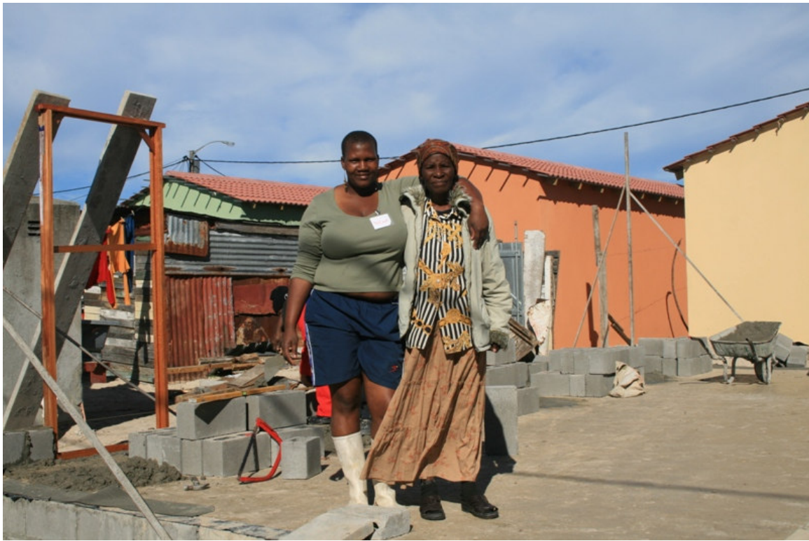
Beneficiary Nolizwe Ntibane and her mother Nokiliva assisting at the construction site of their new home.
