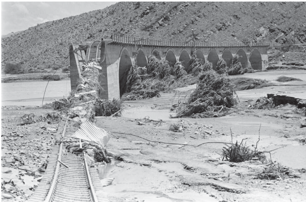
Damage sustained by the railway bridge following the 1981 Laingsburg floods when the Buffels River flooded, claiming more than 100 lives.
