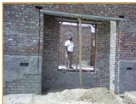
◀ Lubabalo Dzedze inspecting the construction of Leeu-Gamka Library in Beaufort West Region
