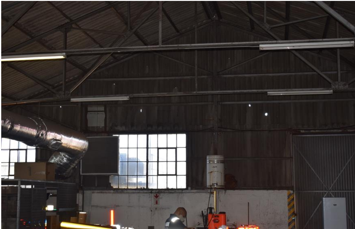
Image 6: Damaged to the side structure of factory caused by children.
