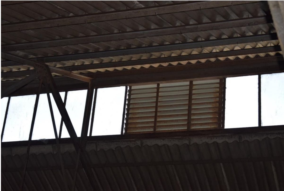
Image 2: Damaged roof with several holes and is the south side of the building.
