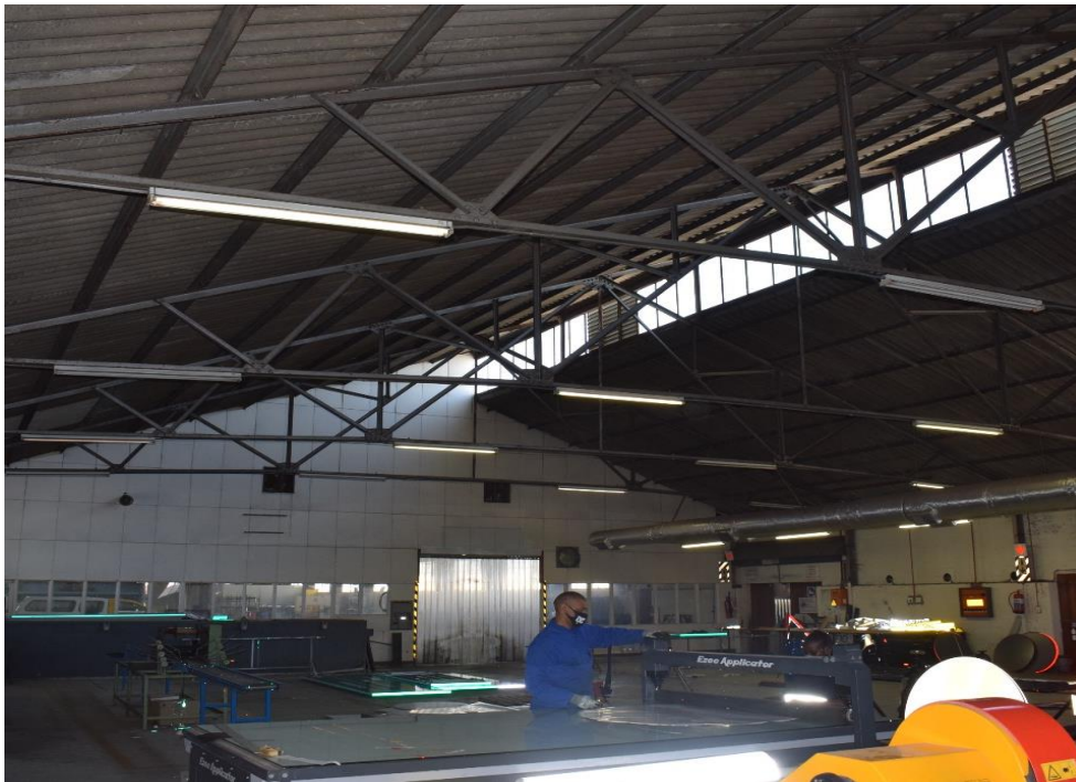
Image 3: Shows the burst light bulbs on both sides of the factory.
