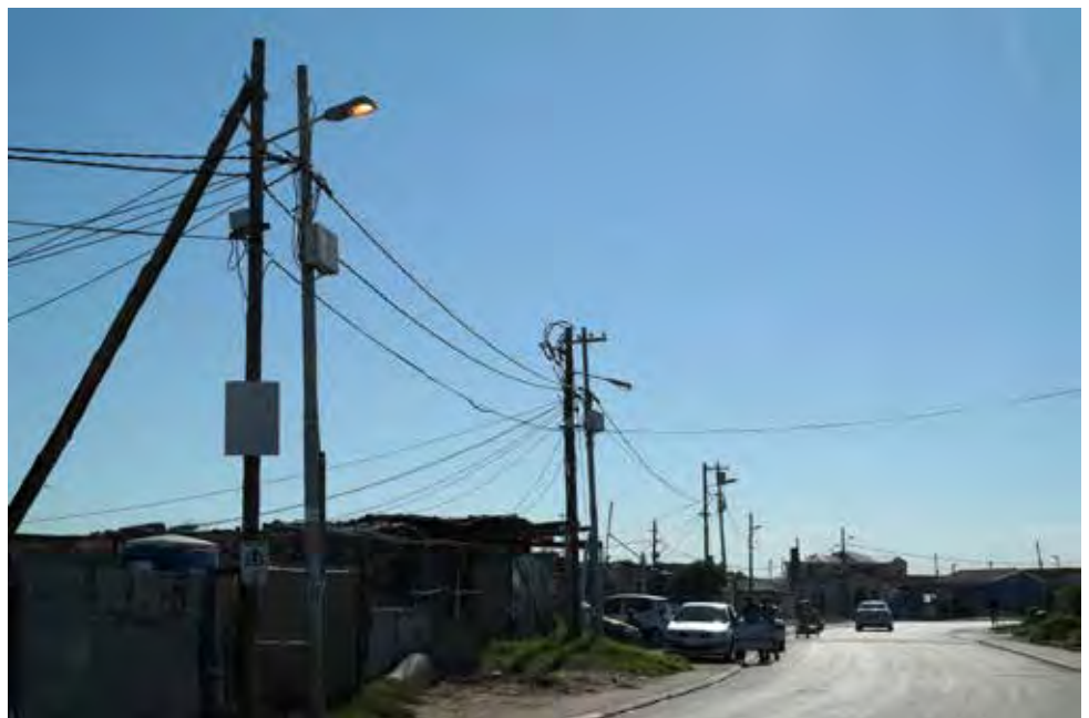
Switched on street lights in KTC
