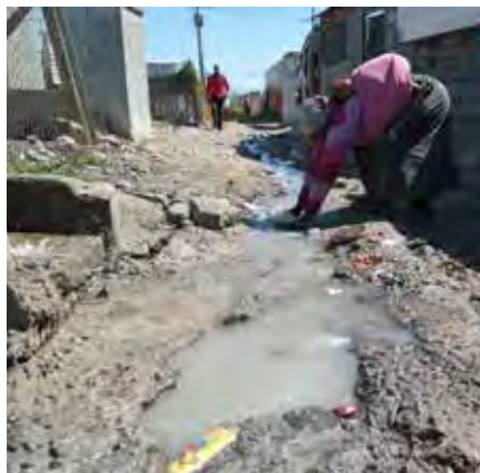
Inadequate drainage in Kosovo
