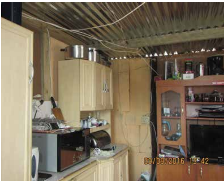
Figure 20: Overloading of electrical circuits in an informal dwelling
