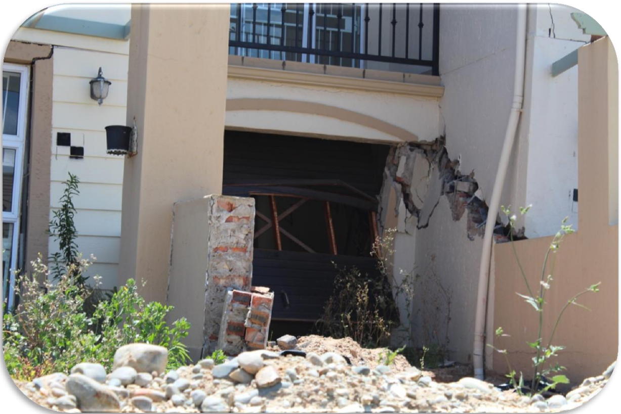
Damaged house in Seemeevlug
