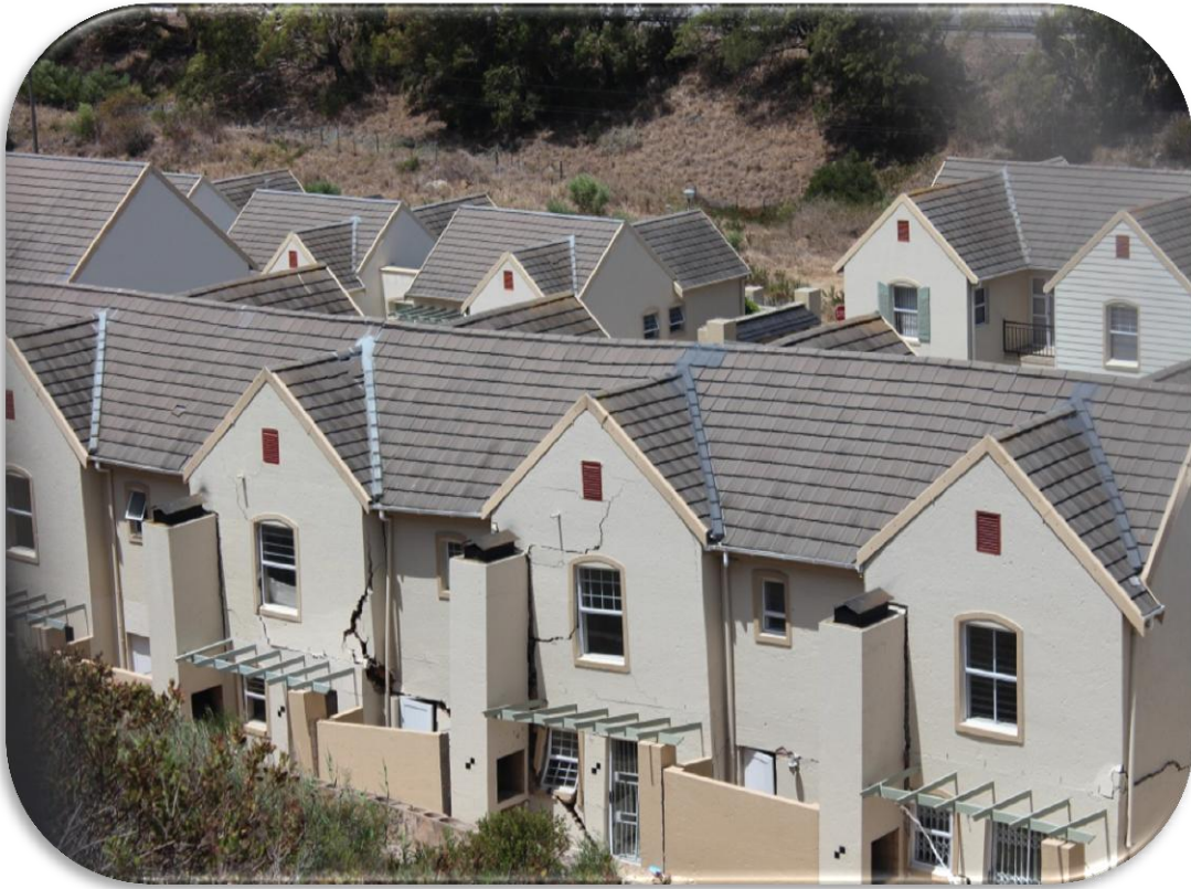
Damaged houses due to the Landslide: Tuscan Village
